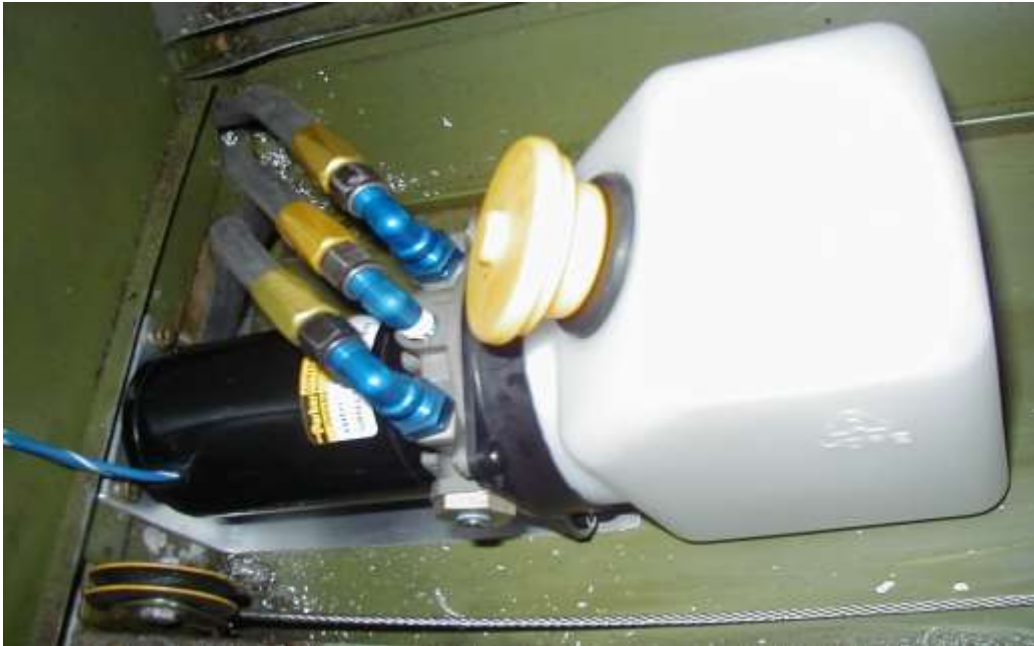
Electric Pump Mounting -Photo 5
